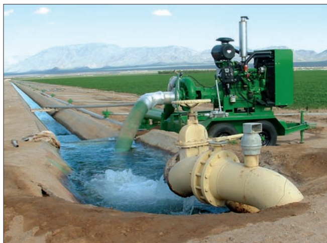
Ground water is withdrawn for irrigation.
