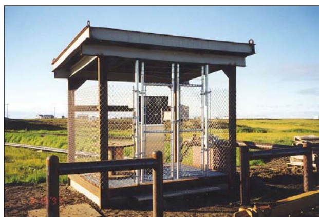
Figure 3-2. Fencing around a dispenser pump.
