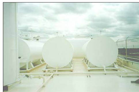
Figure 7-3. Shop-built containers elevated on saddles.
