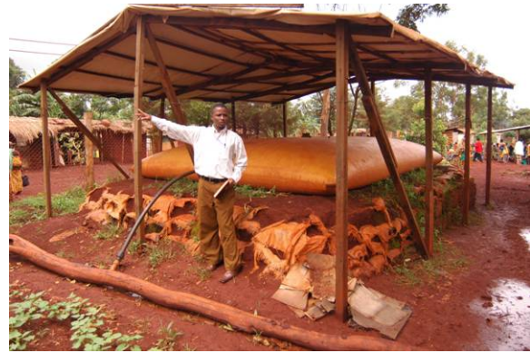
Water storage bladder at Mtabila II Dispensary
