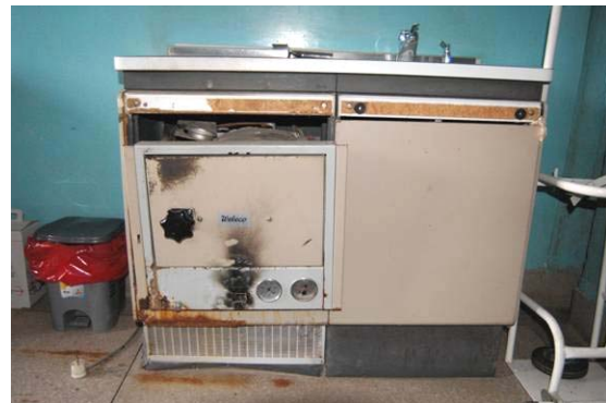
Burned out autoclave
