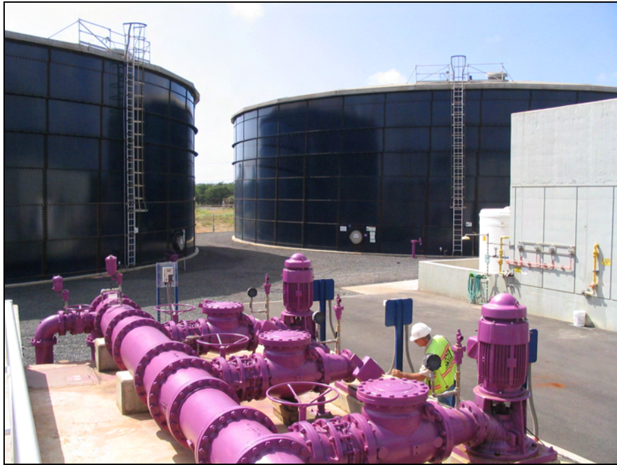
The Honouliuli Water Reclamation Facility produces both R-1 and R-O recycled water. The Honolulu Board of Water Supply has integrated recycled water into its overall water conservation plan.
