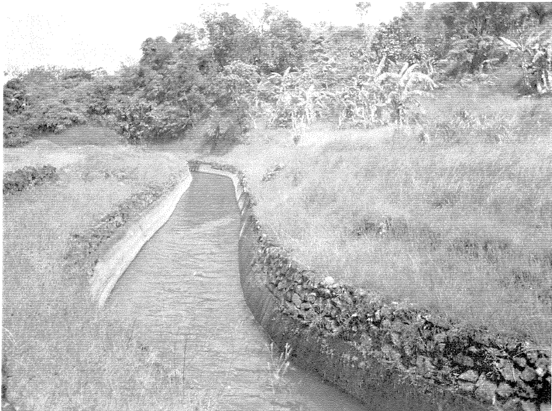
Plate 42B. Koolau ditch in the Nahiku area, East Maui. Photo by Ray Baker.
