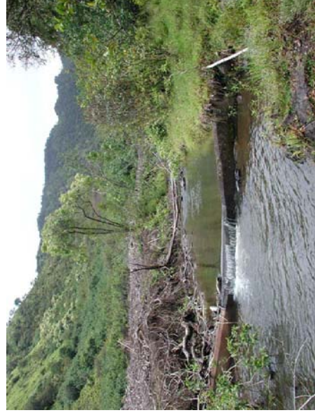
Upstream view of concrete dam on Waiokamilo Stream showing areas where the hau, Hibiscus tiliaceus , are cut back.
