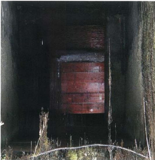
Number 11 intake with board gates to let waterfall flow downstream across the roadway.
