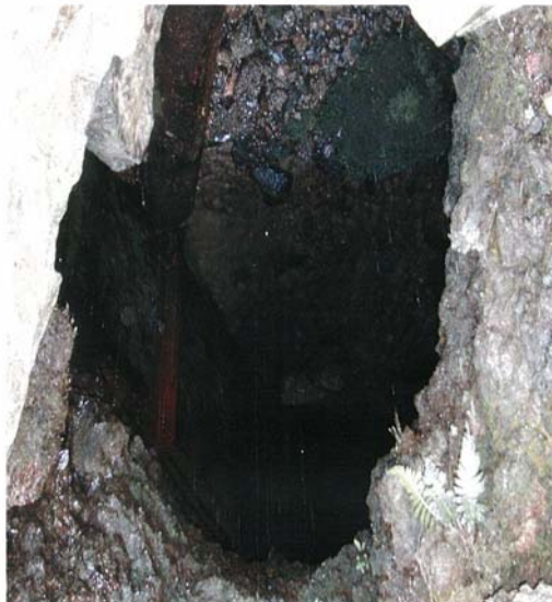
Number 11 intake to tunnel without the board gates, allowing the water to flow back into the Koolau Ditch.
