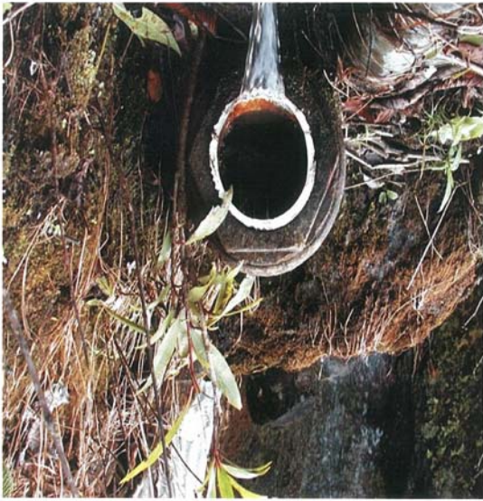
Number 12 intake pipe with the 4-inch PVC cut away (looking upstream).
