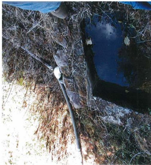
A 2-inch intake with a drisco line leading to a larger pipe.
