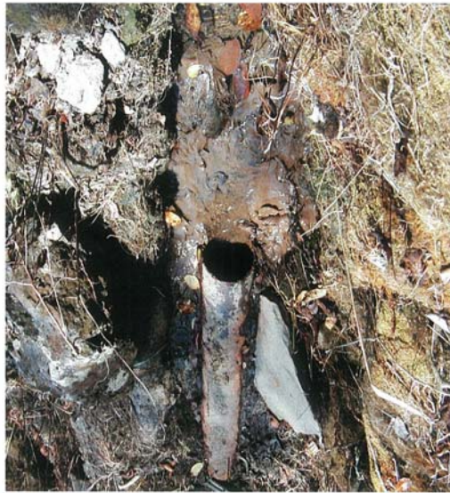
Number 12 pipe intake above the third ladder (looking downstream). This pipe leads to a 4-inch PVC pipe that flows to the Number 12 intake window.
