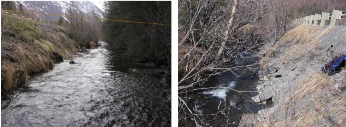
Figure 9. The Lower Highway Reach of Daves Creek. Note the erosion along the highway embankment and the lack of floodplain.
