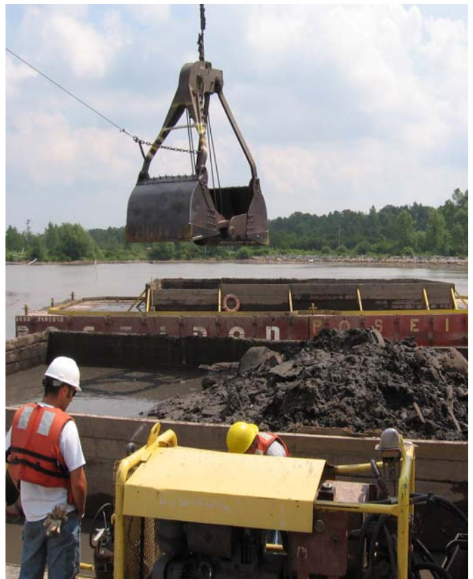
A dredge deposits sediment dug out of Tannery Bay onto a barge. Workers removed the water from the mud, treated the water and disposed of the contaminated materials.
