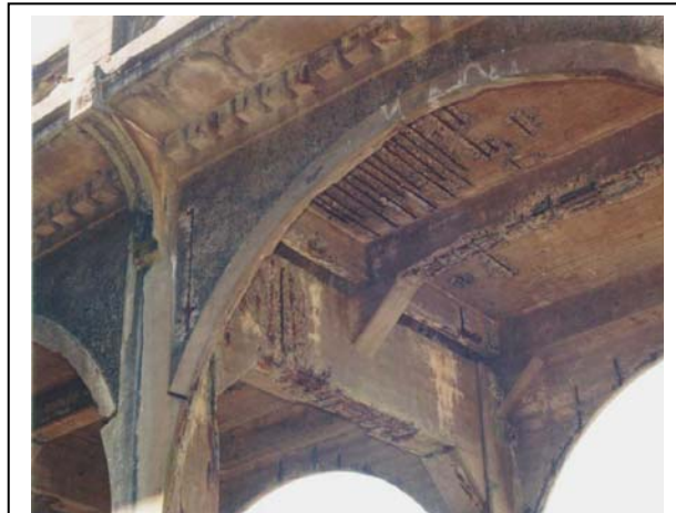
Structural deficiencies on the deck affect load capacity on the 76-year-old Old Winchester Bridge. (North Umpqua River in Douglas County)
