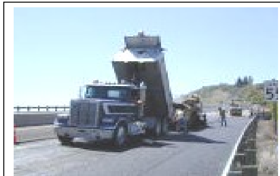
ODOT analyzes pavement deterioration and plans for future improvements.
