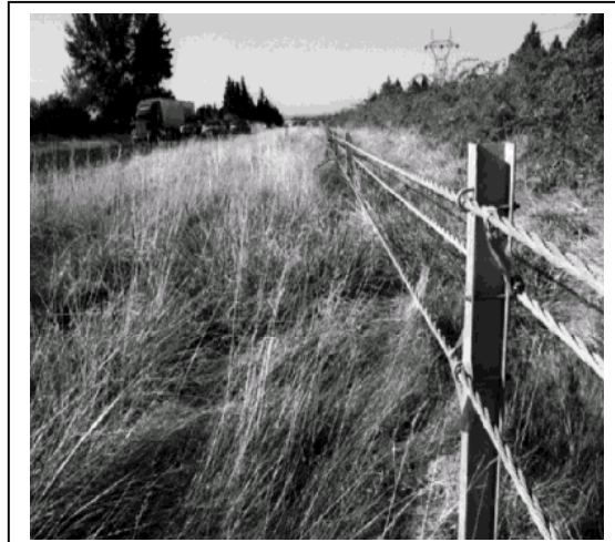
Crash statistics helped pinpoint where to install a median cable barrier along I-5 north of Salem.
