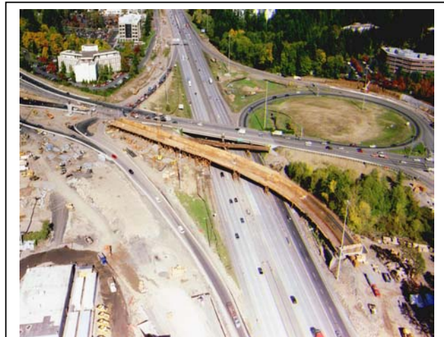
Aerial view of the I-5 and Oregon 217 Interchange redesign. Work on the $36 million project will be completed mid-2001.
