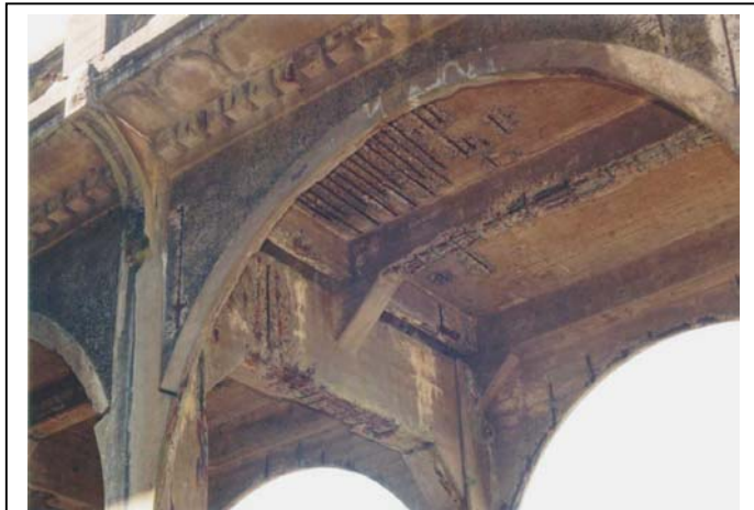
Structural deficiencies on the deck affect load capacity on the 76-year-old Old Winchester Bridge. (North Umpqua River in Douglas County)
