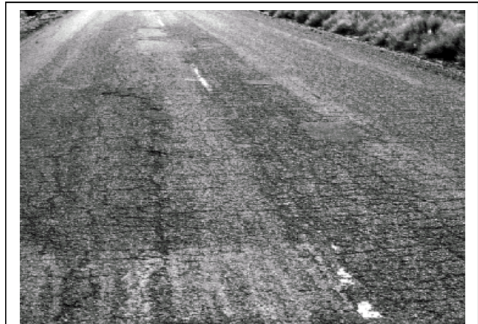
Pavement Condition: Poor
