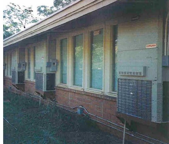
Figure 3.08 - Individual Terminal Units
