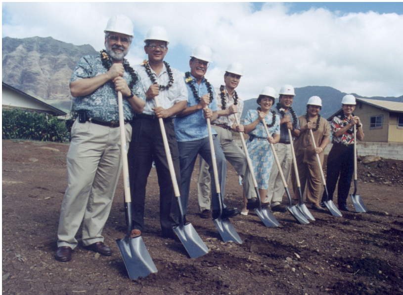
Figure 4. Ground is broken in Wai‘anae for the first energy-efficient Model Home on November 6, 2000 by representatives of cooperating businesses and agencies. Pictured (left to right) are: Peter Dreyfuss, Deputy Chief of Staff, Energy Efficiency and Renewable Energy, USDOE; Raynard C. Soon, Chairman, Hawaiian Homes Commission; Chuck Ehrhorn, AIA, President, Honolulu Chapter, American Institute of Architects; Maurice H. Kaya, Program Administrator, DBEDT ERTD; Audrey Hidano, President, Building Industry Association of Hawai‘i; Randy Lau, Owner, Designer Built Systems; Jackie Mahi Erickson, Vice President, Hawaiian Electric Company, Inc.; Terris H. Inglett, President and Chief Operating Officer, Honsador Lumber Corporation.
