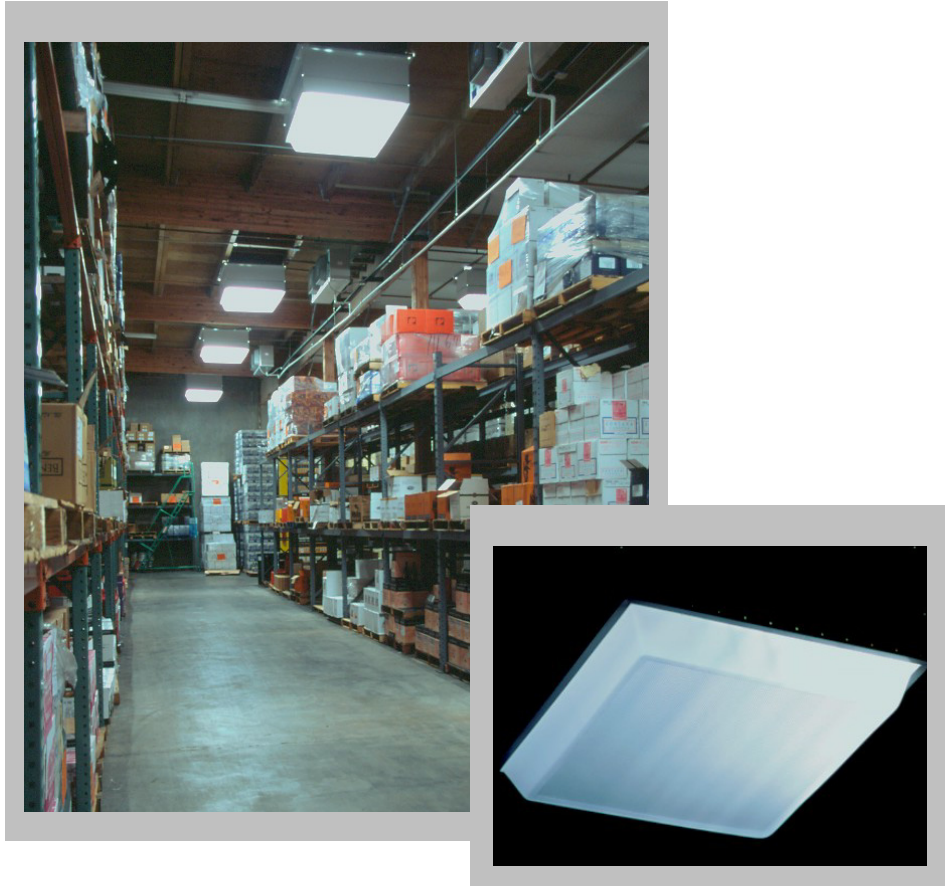
Figure 3-26. Better Brands warehouse, Oahu. Skylights with integrated light wells, fluorescent lighting, and diffusers (inset). Photos: Erik Kolderup, Eley Associates.
