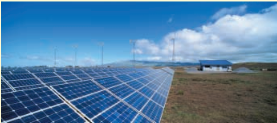
The 225 kW PowerTracker/Wind Hybrid System , designed and built by PowerLight Corporation for Parker Ranch.
