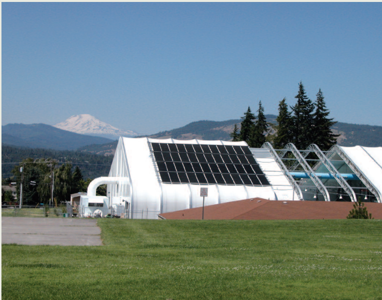
The aquatic center in Hood River has a nearly 5,000 square foot solar hot water system to heat a 281,000 gallon pool. Retractable panels open in summer.
