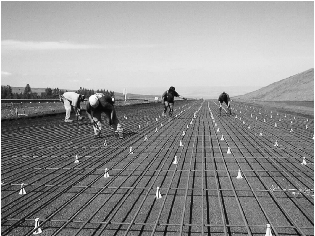
Crews are adding a lane to a segment of Interstate 84 on Emigrant Hill near
