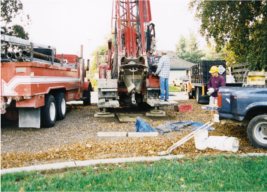
Figure 21. Drilling and installation of a new monitoring well in the Sacramento metropolitan area. This study of shallow ground water was the first of its kind within the Sacramento metropolitan area.
