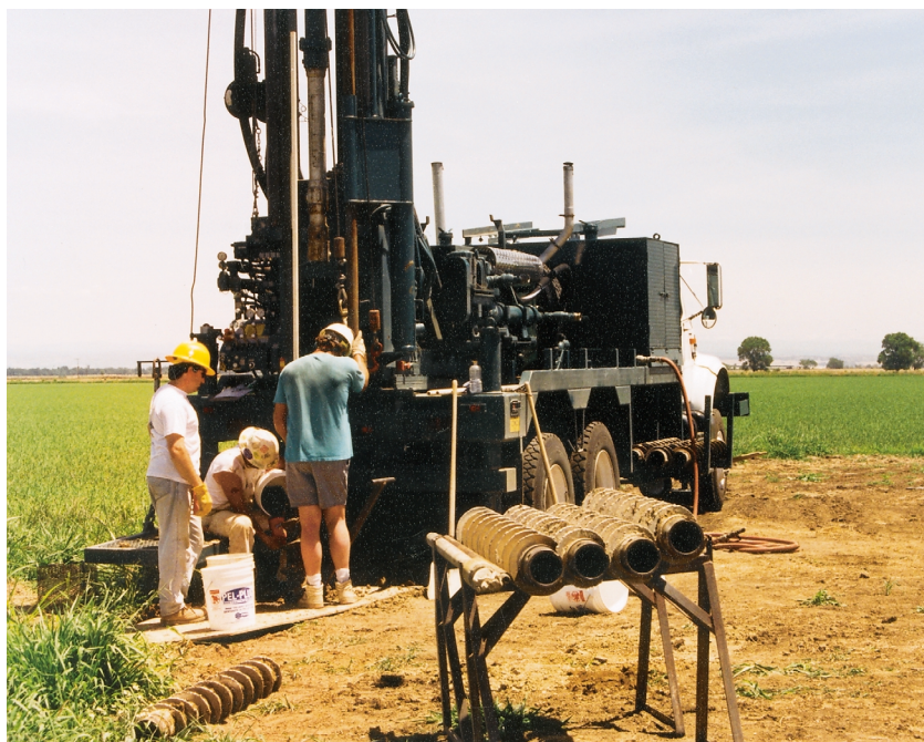
Figure 20. Drilling and installing a new monitoring well in the rice-growing region of the Sacramento Valley.
