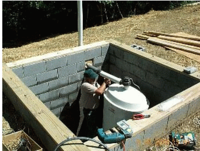
Figure 20. Aeration system and holding tank.
