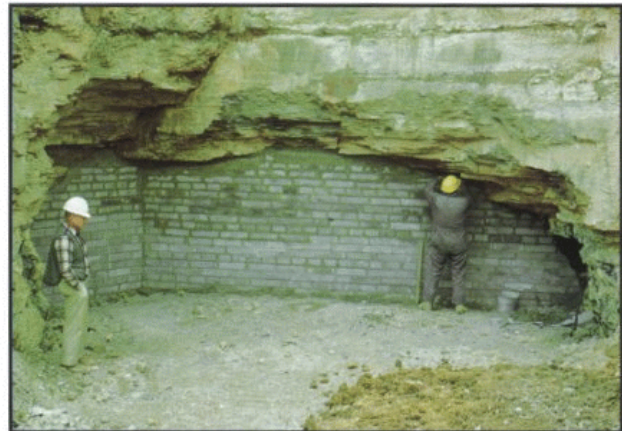
Figure 17. A concrete block dry seal placed at an abandoned mine land reclamation project in West Virginia. (West Virginia Division of Environmental Protection).
