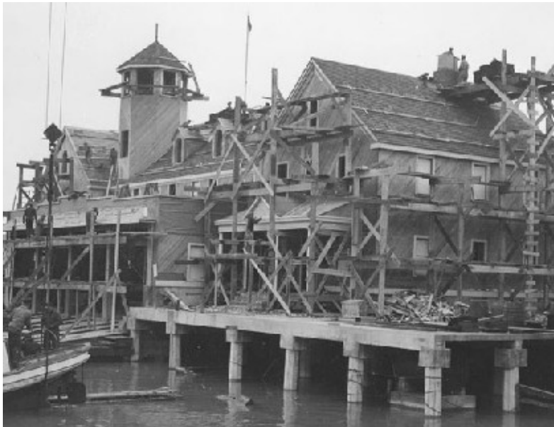
Original photo caption: "Old Chicago Station [;] West & South Elevations - Taken from S.W."; photo was dated 13 November 1935.
