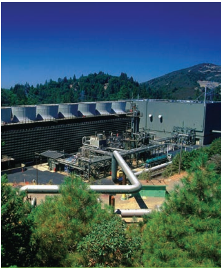
Geothermal energy plant at The Geysers near Santa Rosa in Northern California, the world's largest electricity-generating geothermal development. Photo from Calpine Corporation, NREL/PIX 17270
