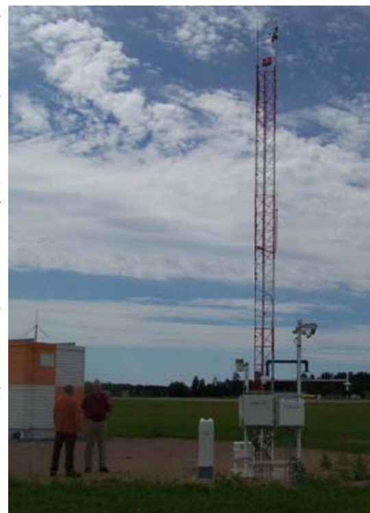
Grand Forks NWS Aviation Program Leader, Dan Riddle, talks with Bemidji Airport Manager, Harold Van Leeuwen, at the base of the KBJI Automated Weather Observing System (AWOS).
