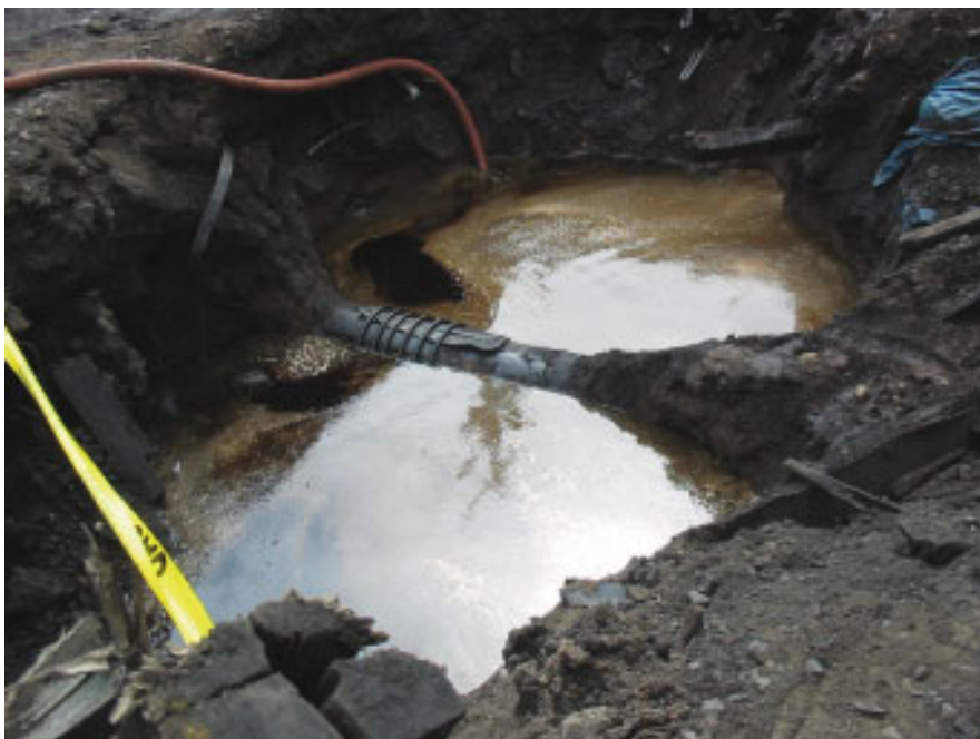
Buckeye Pipeline Rupture
