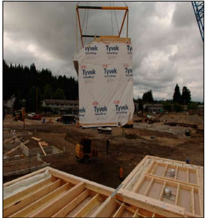
A crane lifts the modular units in place. The units are built at the Champion factory in Silverton, Oregon and transported to Fort Lewis.
