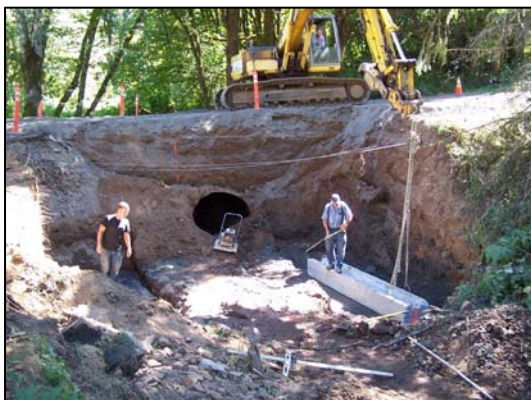
Figure 4a. Sample opportunistic photo documenting the installation of a new culvert providing upstream fish passage (Scappoose Watershed Council).
