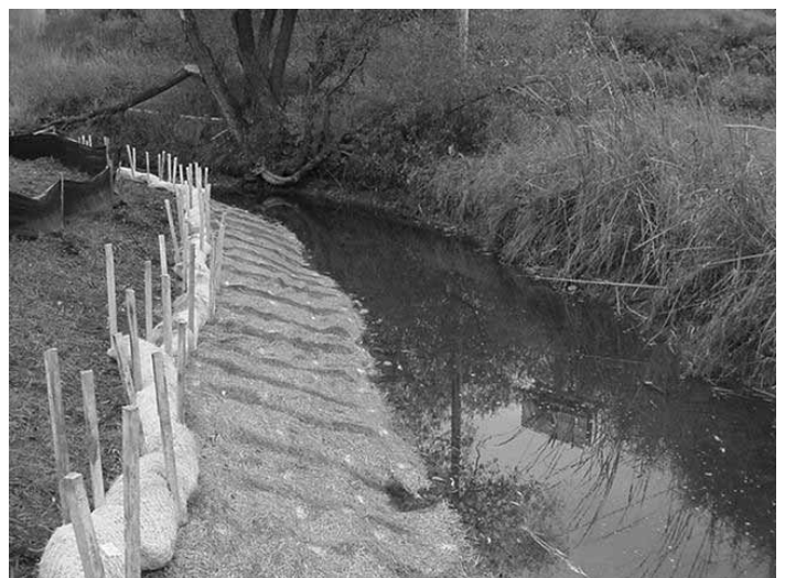
After contaminated sediment was removed from Newton Creek, the banks were stabilized.
