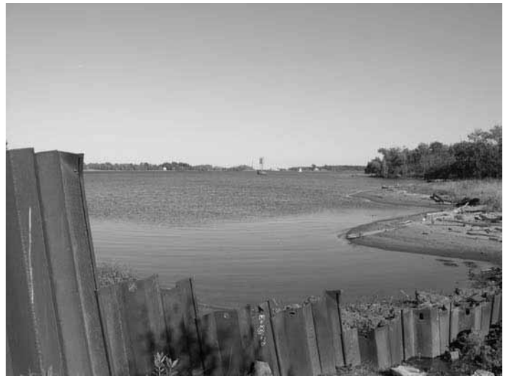
Sheet piling kept water from Superior Harbor from reflooding Hog Island Inlet.
