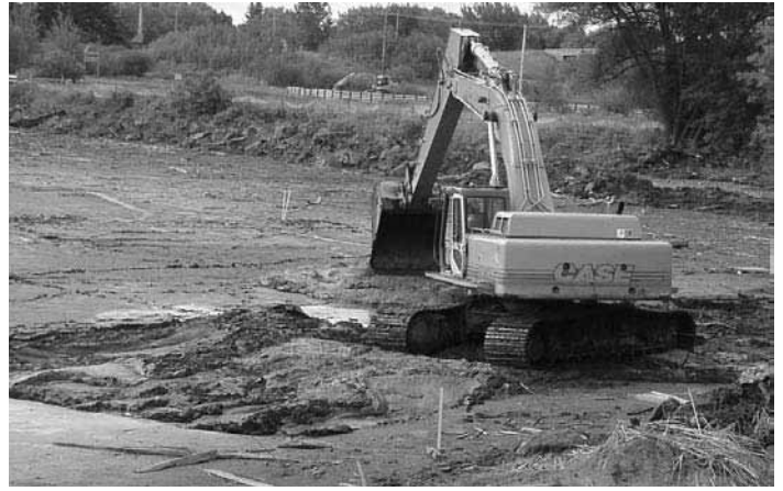
After water was pumped out of the inlet, sediment was excavated with traditional construction equipment.
