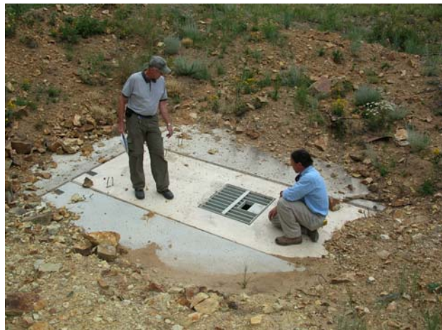
Pre-cast concrete panel closure with locking access door over vertical opening GG-23 of the Gilson Gulch noncoal project
