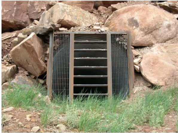
Bat grate in corrugated metal pipe closure in portal at Shelby Dean site of Mesa State College noncoal project
