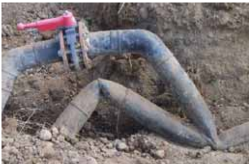
Figure 11. LFG Pipe Buckling Failure
