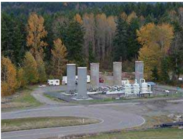
Figure 9. Blower/Flare System at Cedar Hills Regional Landfill
