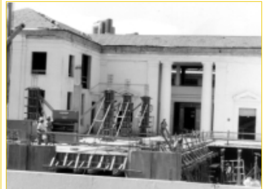
Renovating the Carnegie Library took nearly two years to complete. The library’s expansion took place at the rear of the building, more than doubling its size from 47,000 to 102,000 square feet.
