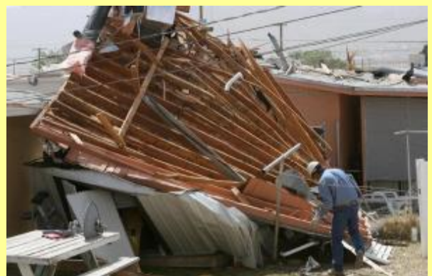
Wind gusts around 50 mph tear a roof from a building in El Paso on April 10. (Mark Lambie El Paso Times)
