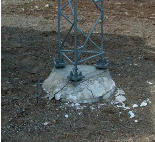
Aging tower base at Halfway Hill site
