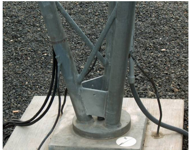
A well-grounded, well-constructed tower base at the Whitmore Rd. site
