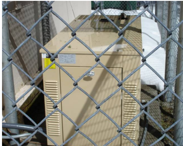
A secured, modern generator at Mt Whitmore
