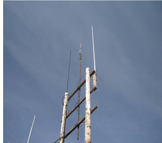
Radio antennas on wooden poles at Nicola Mountain site
