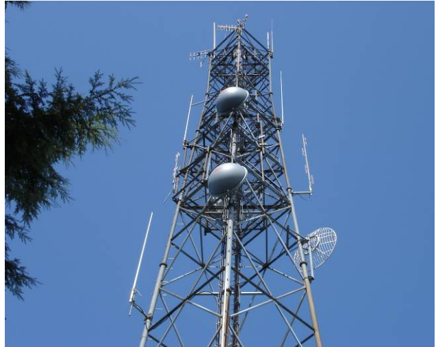
A well-constructed, high-capacity tower at the Table Mountain site
