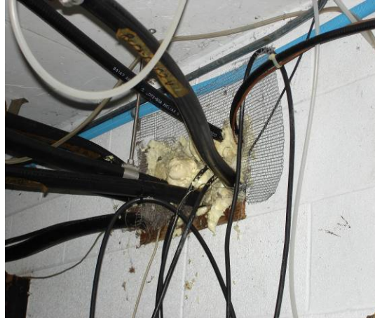
Cable entrance at Baldy Butte site
