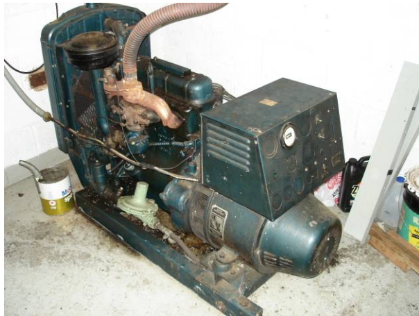
Aging generator at Baldy Butte site
