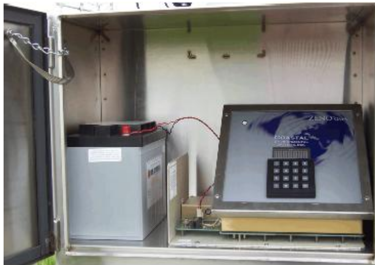
Figure A-16. Data Logger Box
