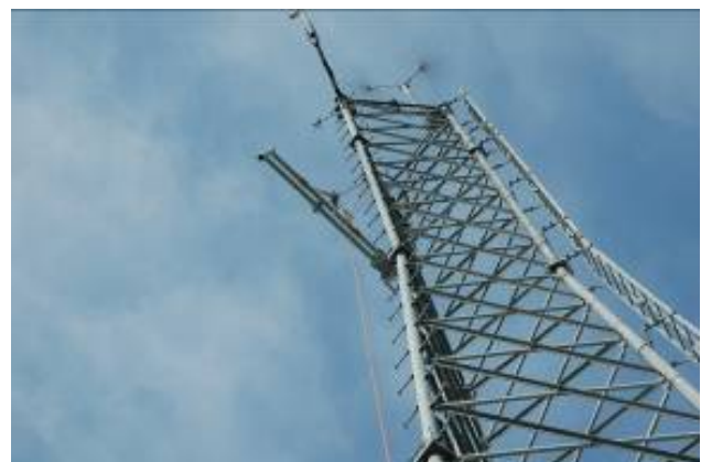
Station Brunswick, GA, tower with NAIS I-1 Antenna installed NAIS I-1 Resource Guide
