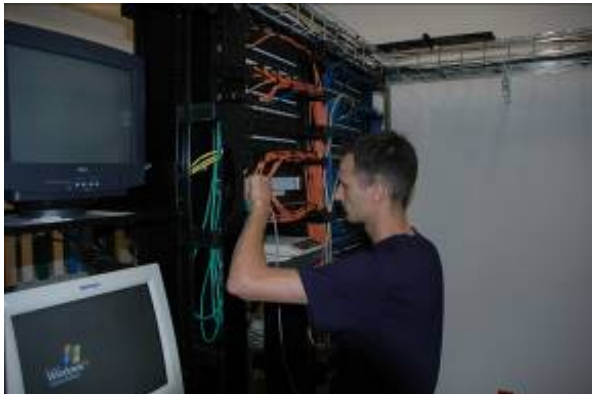
ET2 Spalding from ESD Mayport examining the NAIS I-1 equipment installation
