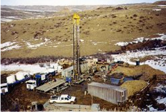
Figure 5. Photo of a Coal Bed Methane Well.
