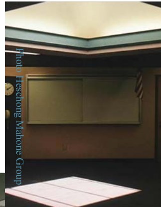
Glare From Skylight
