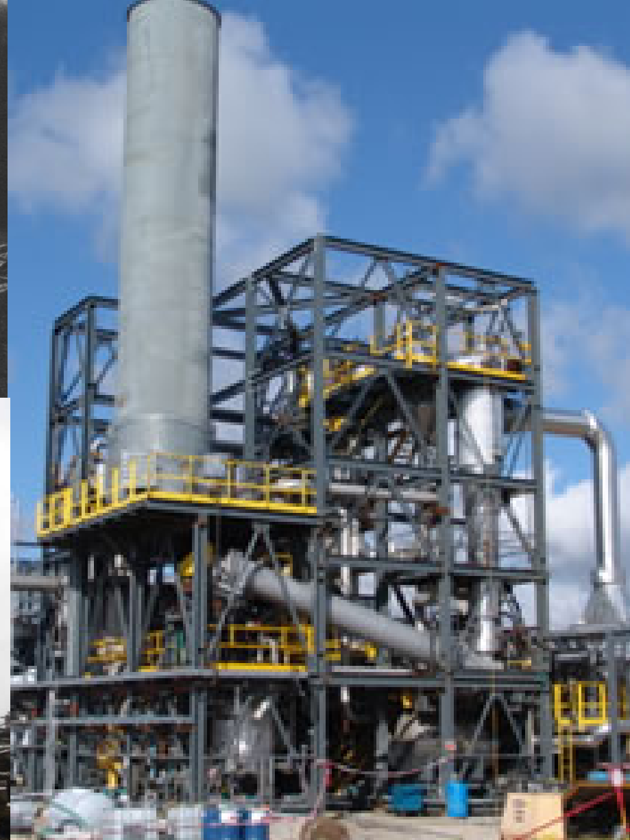
Modern Fast Pyrolyzer Dynamotive Energy Systems Co.
