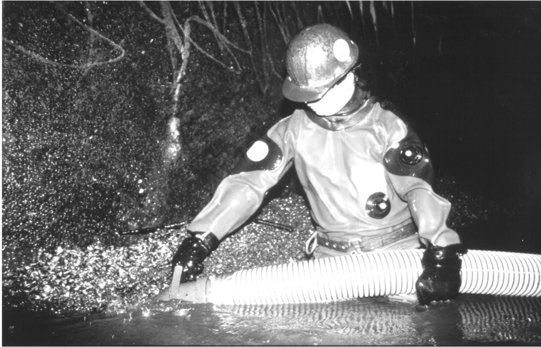
Figure 5. Removal of zebra mussel shell debris by vacuum hose (photographed by Peter Yates)
