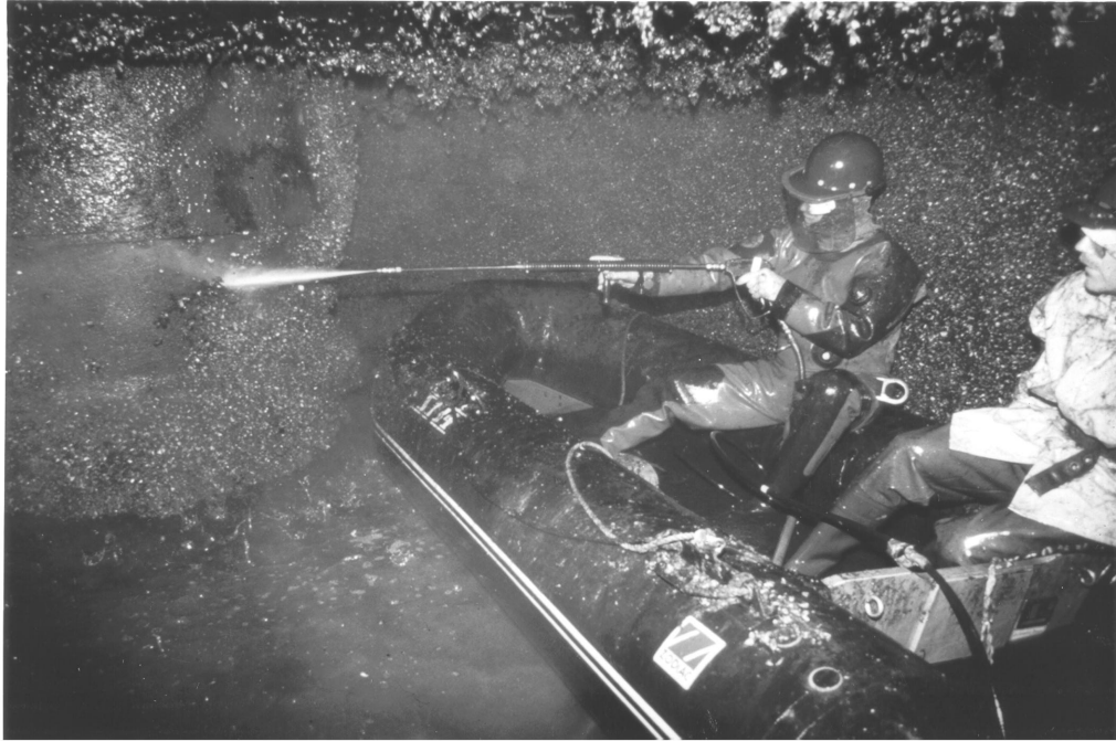
Figure 6. Water jetting being used to clean pump room (photographed by Peter Yates)
