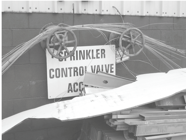
Figure 3-3 Regular Inspection and Testing Should Correct Conditions Like This
