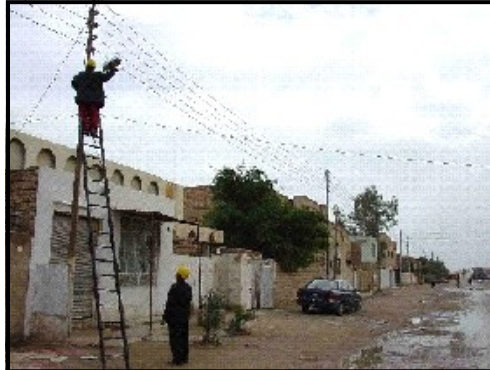
A worker installing a streetlight in in Najaf . This is an example of a Community Action Program project completed in Najaf earlier this year; similar projects are now underway.
