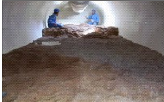
Workers installing a sand layer in a Baghdad water treatment plant sand filter
