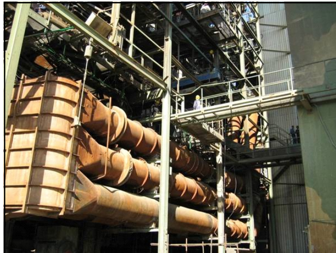
Unit being rehabilitated by USAID in central Iraq; upon the completion of all work, the two rehabilitated units will generate 300 MW
