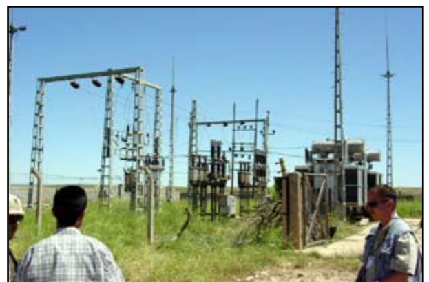
Bechtel assessment team inspects power infrastructure in northern Iraq. (Photo: Bechtel National, Inc.)
