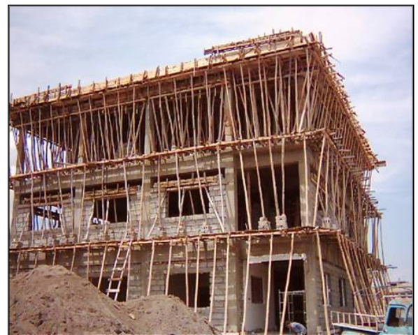
Construction of the new Document Center in Mosul has resumed. The building will house rare documents, some of which date back more than 1,000 years.
