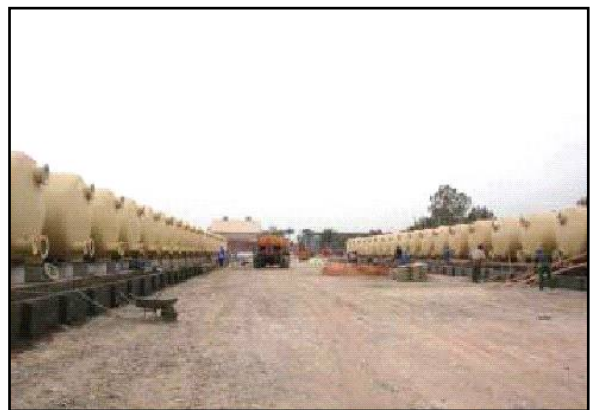
Installed sand filters at Sharkh Dijlah -- Sharkh Dijlah is one of two main water treatment plants that serve 4.7 million Baghdad residents.
