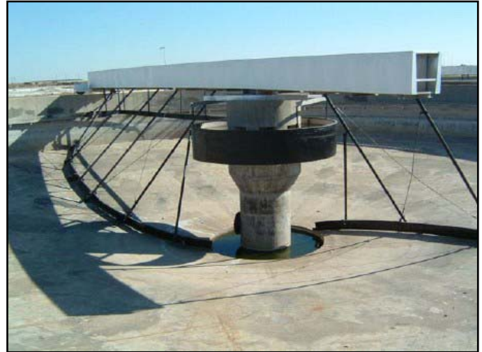
Ad Diwaniyah wastewater treatment plant
