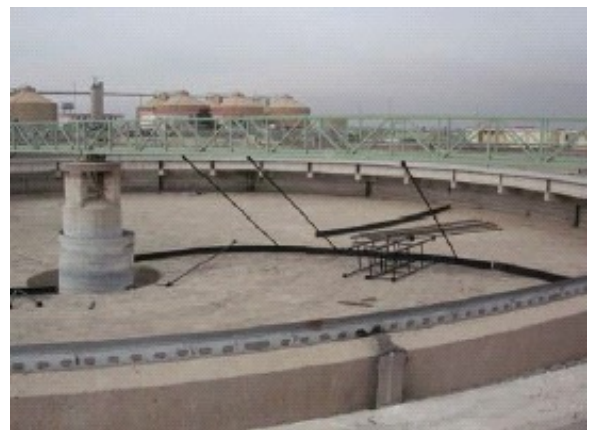
Rustimiyah wastewater treatment plant
