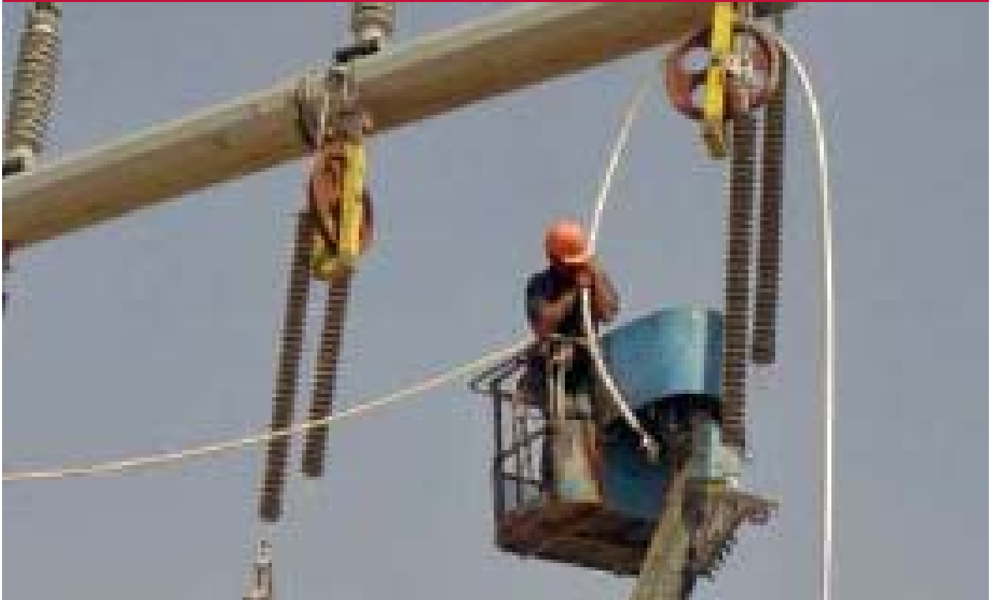
Pulling high-tension switchyard cables at Baghdad South Power Plant. The project will add 212 MW to the national grid when it is complete in July, 2005.
