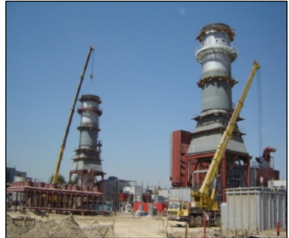
Exhaust Stack External Rings and Silencer.
