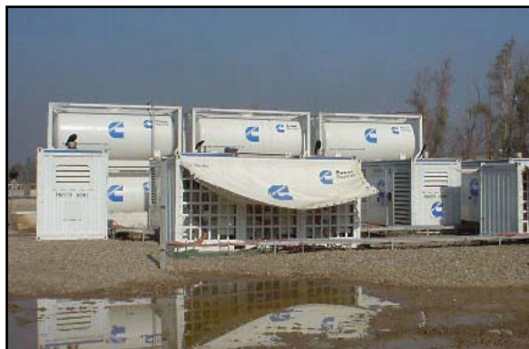
New generation sets awaiting installation at Baghdad International Airport
