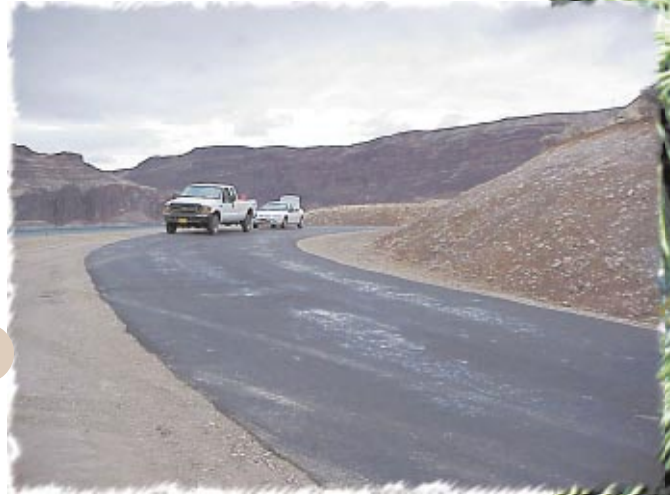
The paving work at Lake Owyhee will provide safer access to the many campers who use the site.
