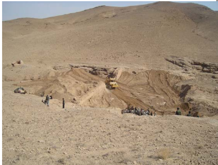
Afghan National Army combat engineers clear dirt and rubble as part of a dam reconstruction project in Zangalan. The project shows Afghans that their new army is capable of more than fighting.
