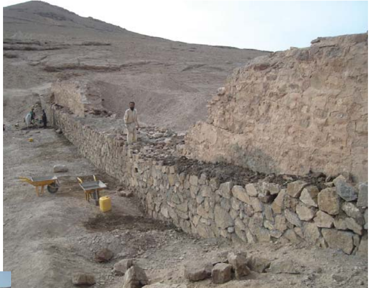
Local contractors work with Afghan National Army combat engineers from 3rd Kandak, 1st Brigade, to reconstruct the Zangalan dam, damaged during the Soviet occupation. This was 3rd Kandak's first real life mission and promises to succeed.
