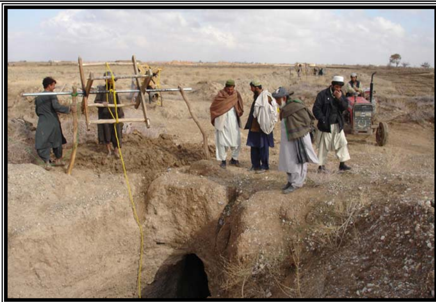
Villagers from Khvosh Ab in Kandahar province work on a karez irrigation system in early January. Much of the repair work was done using methods Afghan farmers have used for hundreds of years.
