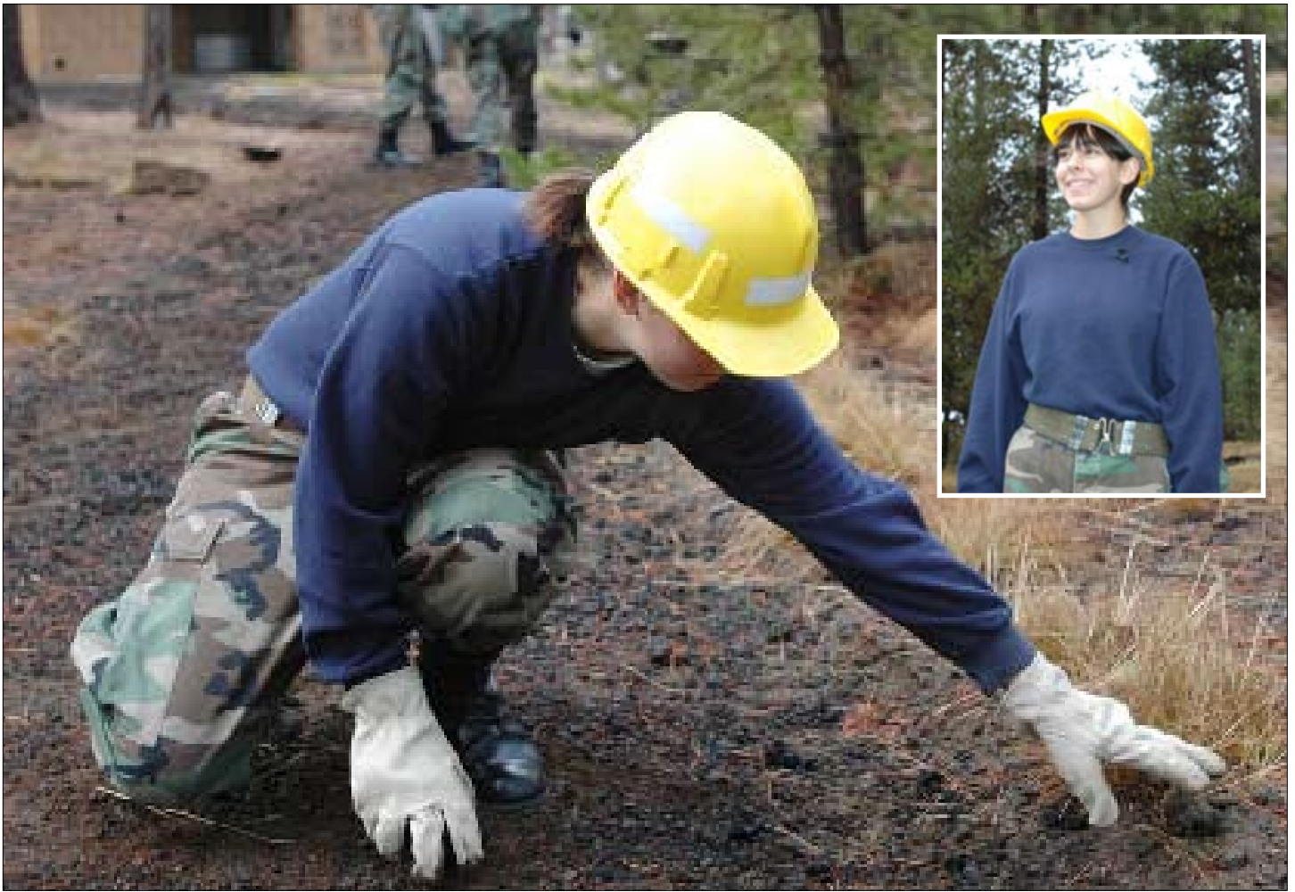
Above: A cadet works to remove asphalt debris in preparation for trail improvements at the La Pine State Park. (Photo by MJ Jacobsen) Inset: Cadet Jasmine Troncoso works hard to improve herself through service-to-community work. (Photo by Spc. Siobhan Gill)
